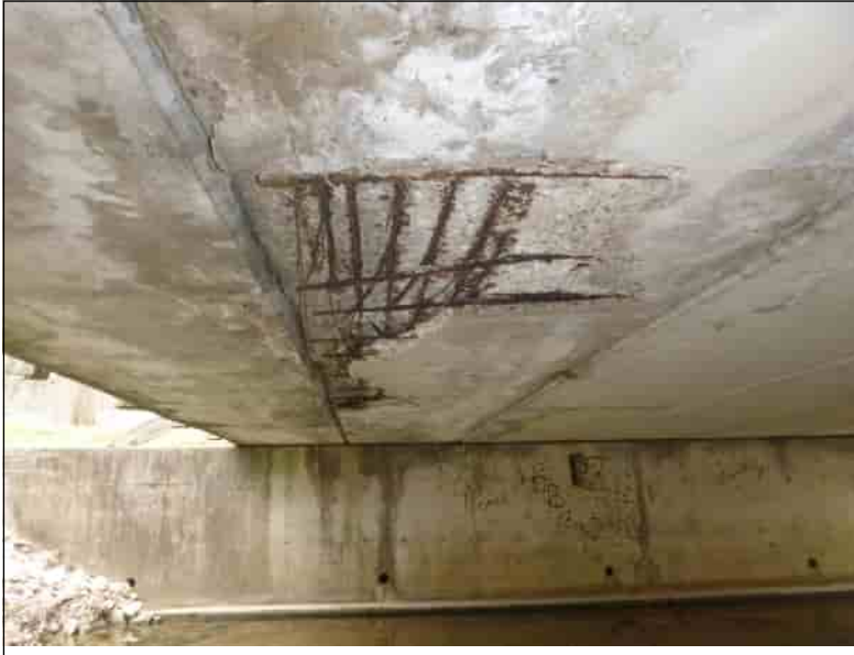
PHOTO #11: ISOLATED MAJOR SPALL WITH 7 SEVERED STRANDS ON BEAM 2 AT MIDSPAN
