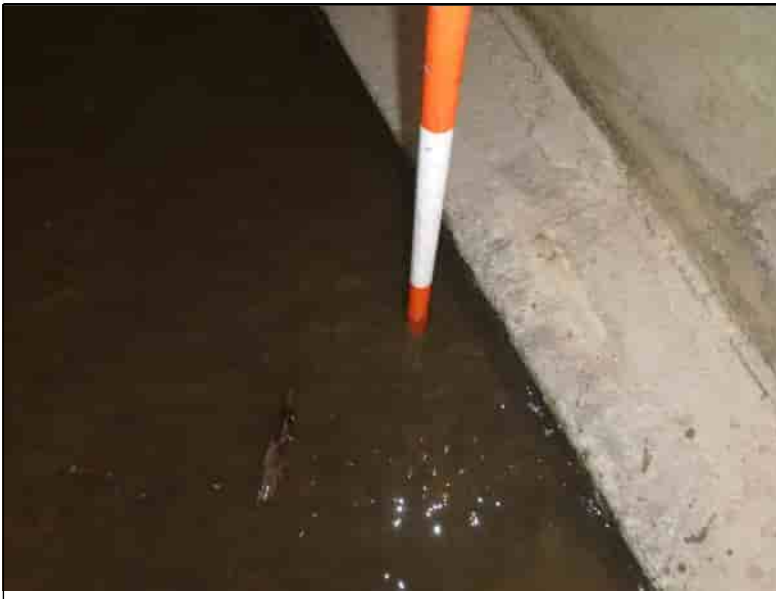
PHOTO #16: 0.8' OF SCOUR AT ABUTMENT 1 FOOTING
