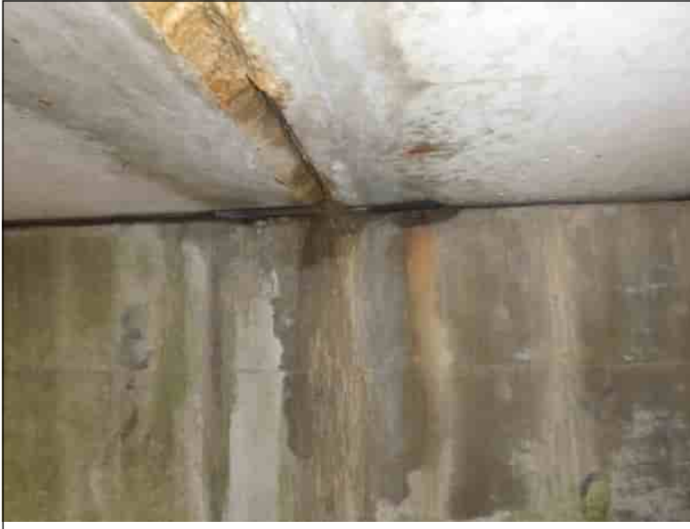
PHOTO #15: ISOLATED MINOR SPALL ON ABUTMENT 2
