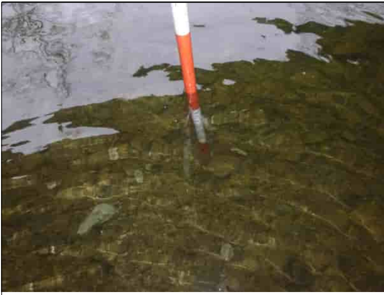
PHOTO #14: SCOUR HOLE AT SOUTH COPING
