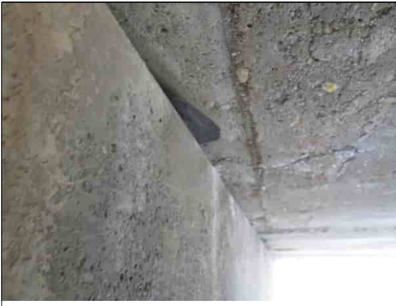
PHOTO #06: TYPICAL BEARING PAD MOVED OUT & OVERHANGS BRIDGE SEAT
