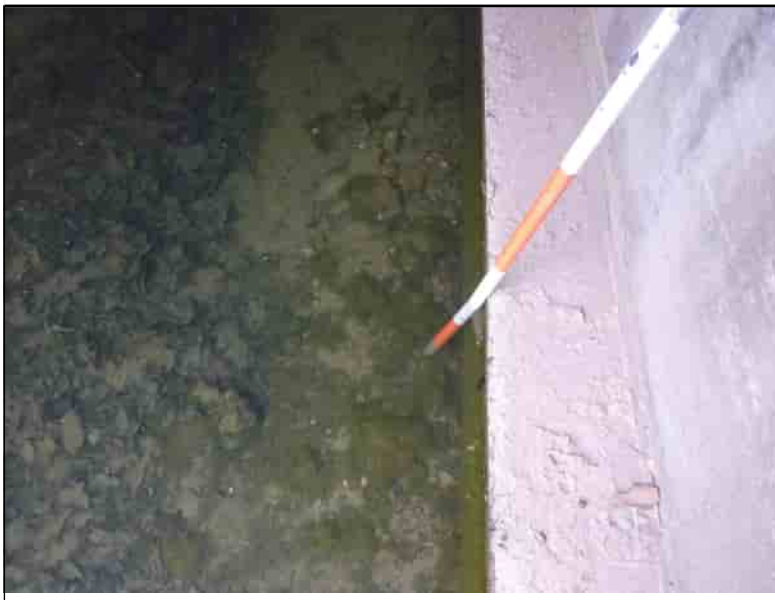
PHOTO #10: 1.5' OF SCOUR AT ABUTMENT 2 FOOTING
