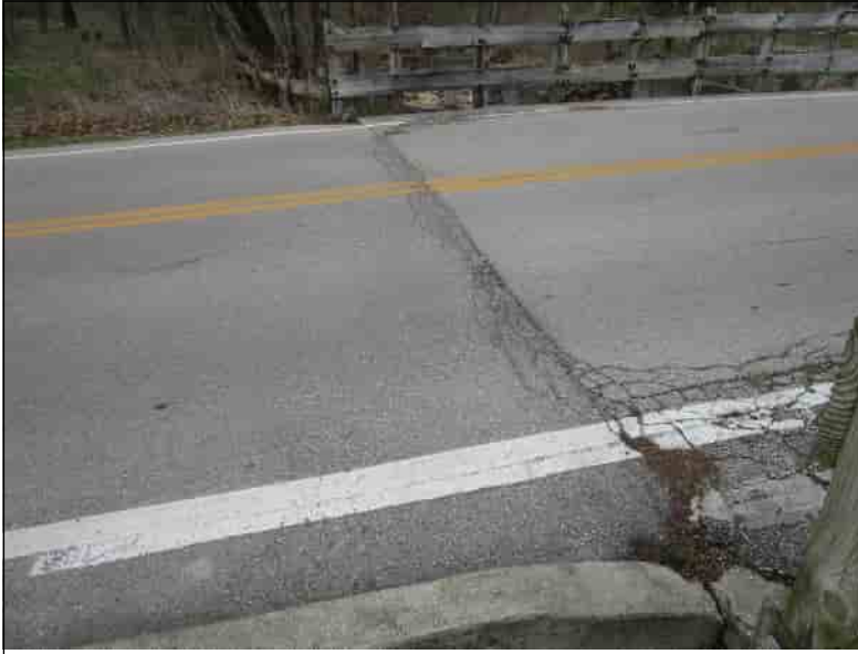
PHOTO #05: ASPHALT CRACKING AT BRIDGE END & ROTTED TIMBER BRIDGE RAIL
