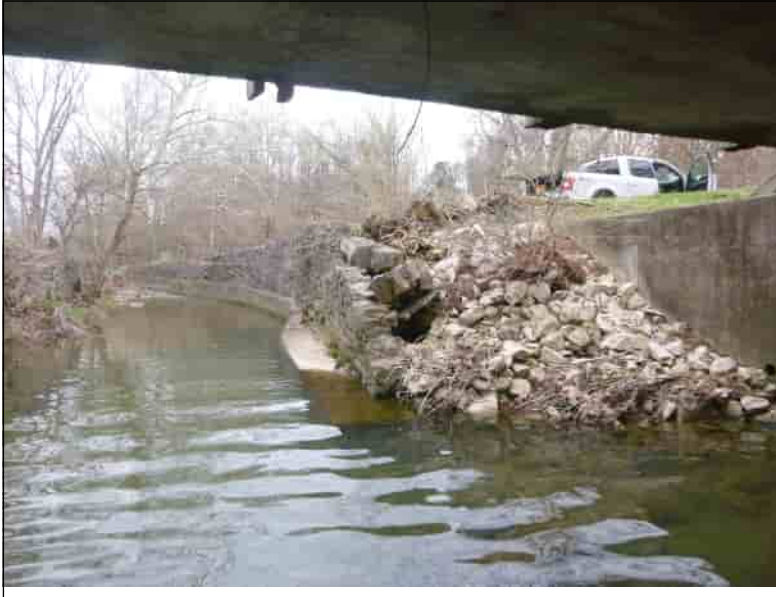
PHOTO #13: SOUTHWEST WING FAILED
