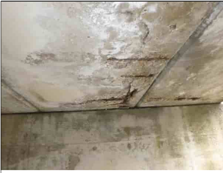
PHOTO #12: ISOLATED MODERATE SPALL ON BEAM 2 AT EAST END
