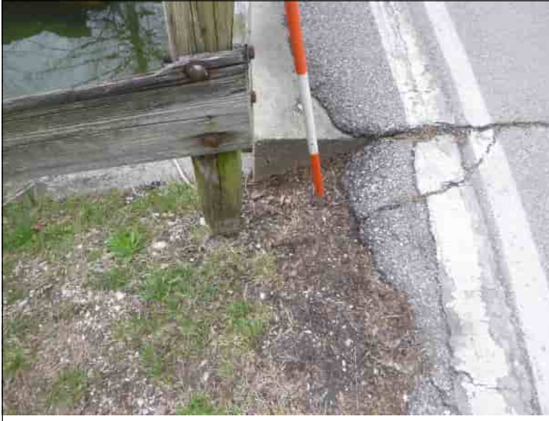
PHOTO #17: MINOR EROSION AT SOUTHEAST BRIDGE CORNER
